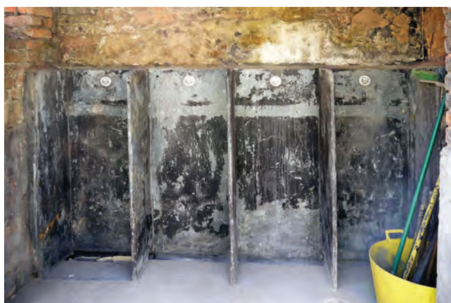
Officers’ urinal block – other ranks would have used much more basic facilities nearby. Photo Clive Penfold
